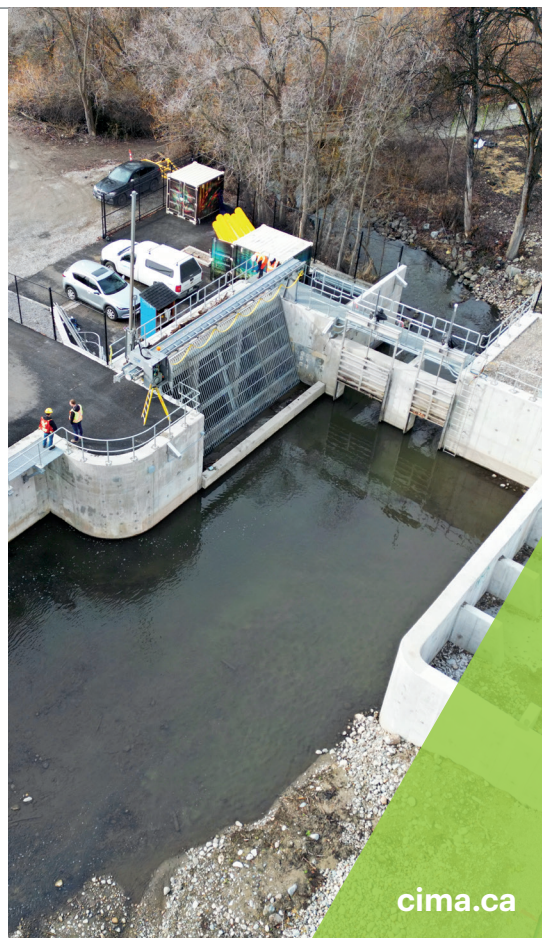
MidSea's Mill Creek intake flood diversion structure City of Kelowna, BC
